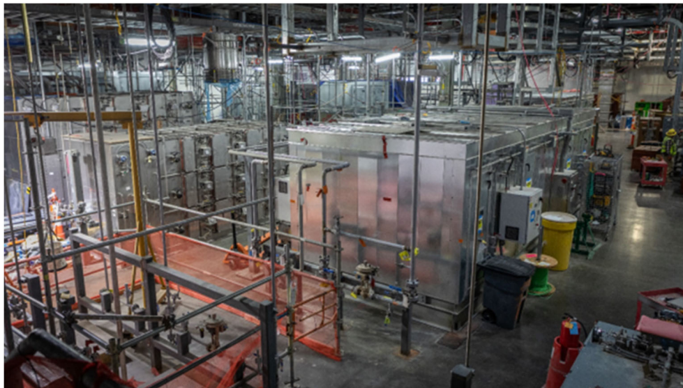
Process equipment installed in the Uranium Processing Facility.
